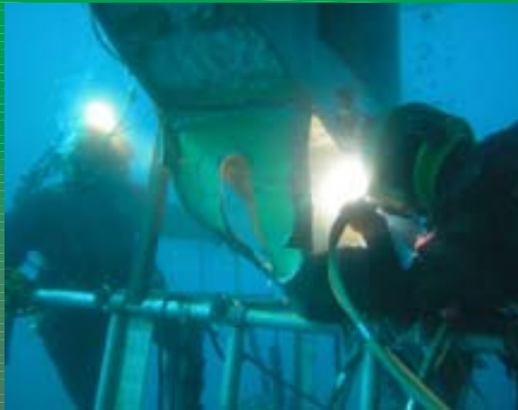
Divers arc gouging damaged stiffener from lower section of rudder.
