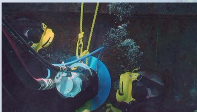
Navy Divers working to position the Underwater Friction Welding System to weld a stud in place.
