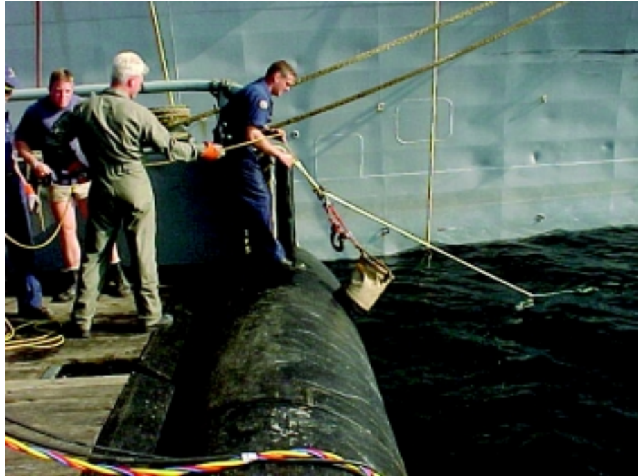
Master Diver Scott Heineman, HTC Mike Lutz, and GM2 Chad Dillon lowering concrete on a trolley line to diver in the water.
