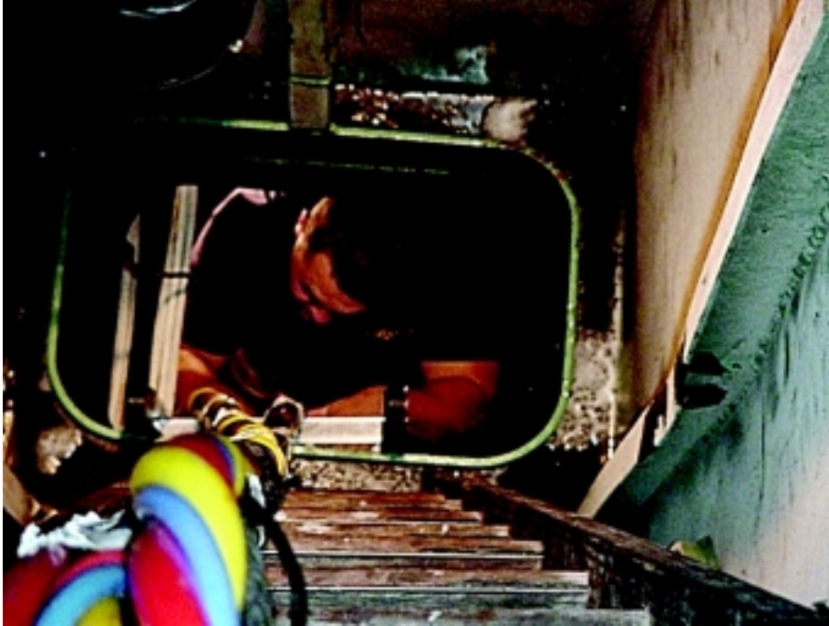
EN2 (DV) Mike Shields routing umbilicals through the engine room vent duct.
