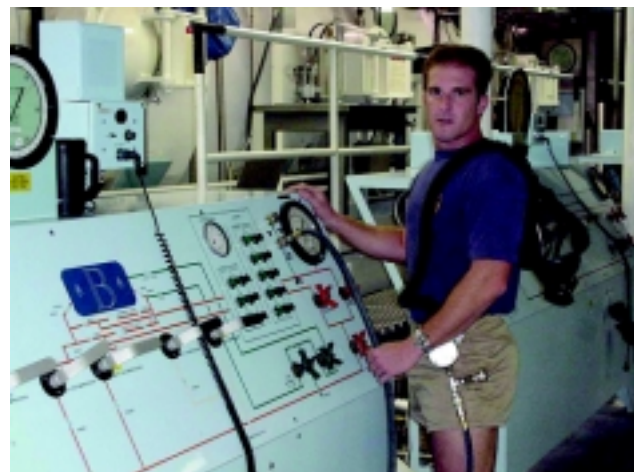
BM1 Larck installing new EBA system at OSF Manual Operating Panel
